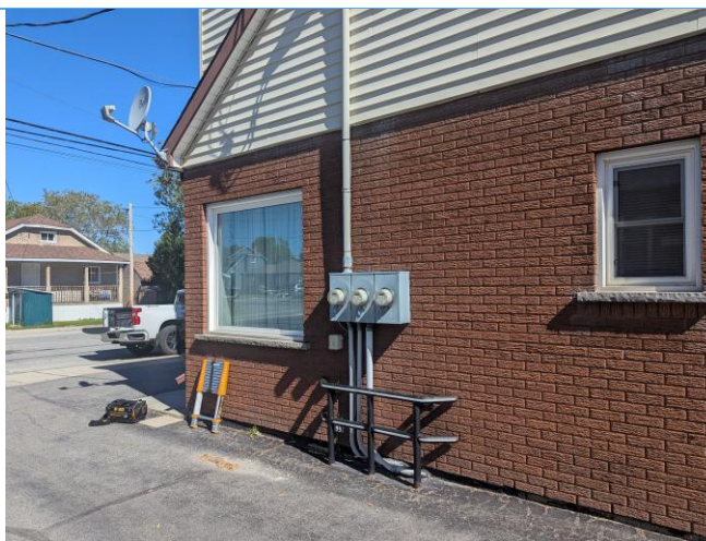
General view of the electrical meter serving the building.
