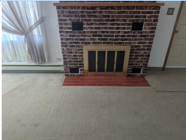
General view of the wood-fired fireplace serving Unit 1.
