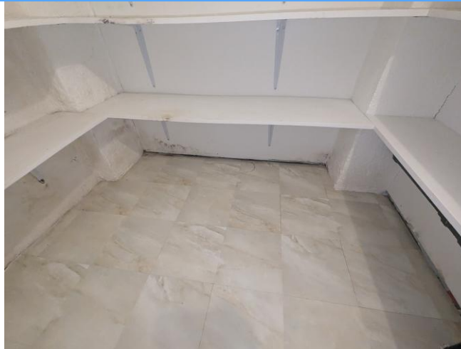
View of the evidence of water infiltration in a cold storage room.
