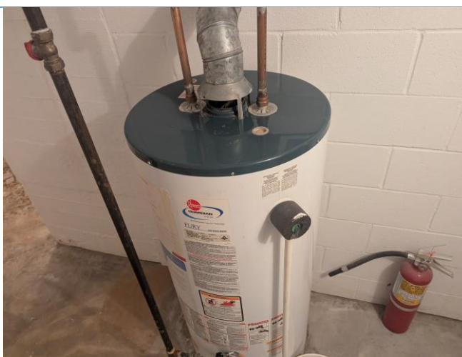
General view of the natural gas-fired "Rheem" DW heater serving the building.
