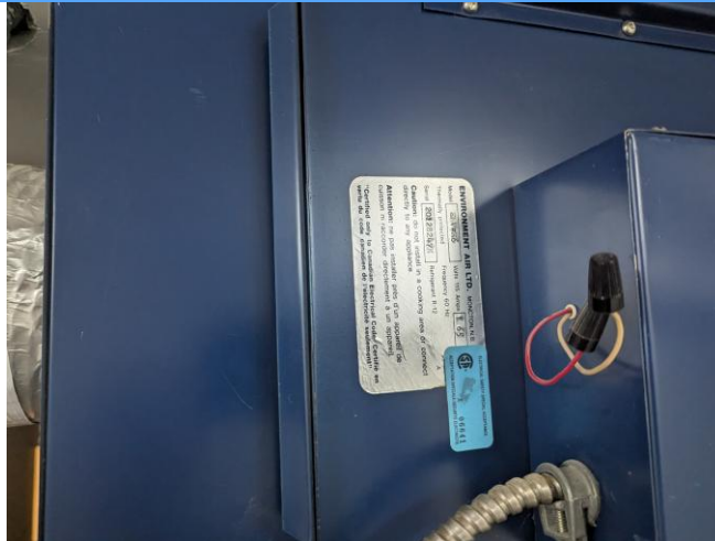
View of the manufacturing tag located on the HRV.
