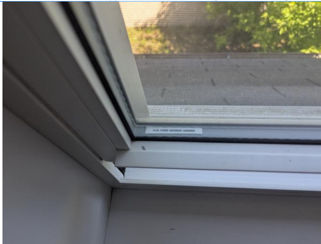
View of the date stamp of ~ 2014 serving the vinyl window of the building.
