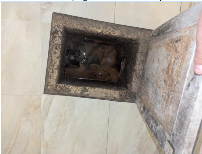
View of the floor drain serving the Site Drainage.
