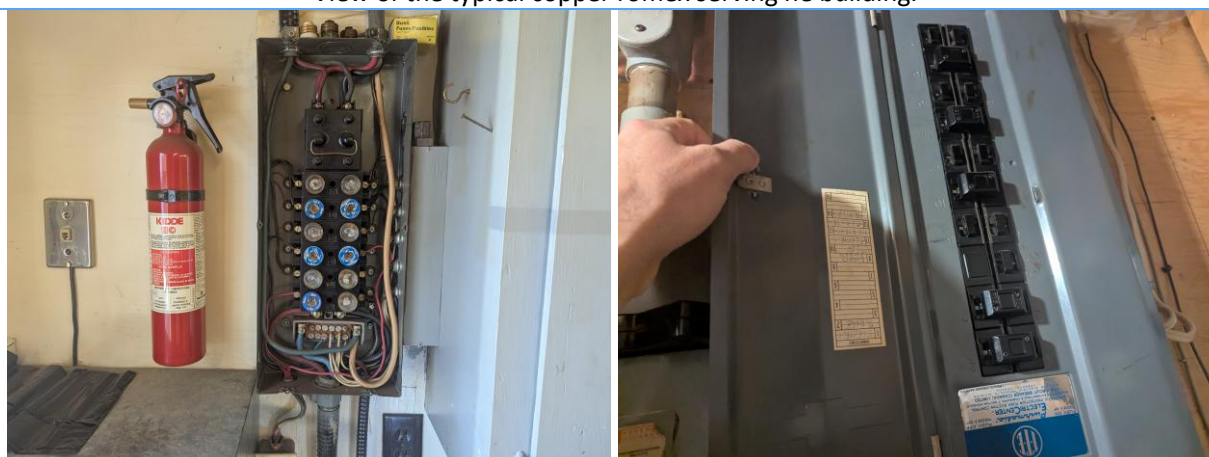
View of the electrical panels beyond their PUL.
