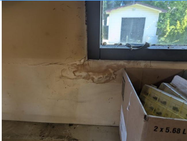
View of the water damage drywall from the leaking window of the garage.
