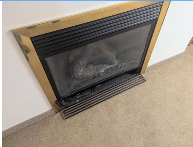
General view of the natural gas-fired "Wolf Steel" fireplace serving Unit 1.
