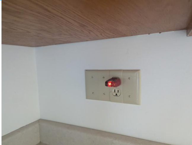
View of the typicla open grounded receptacle serving the building.
