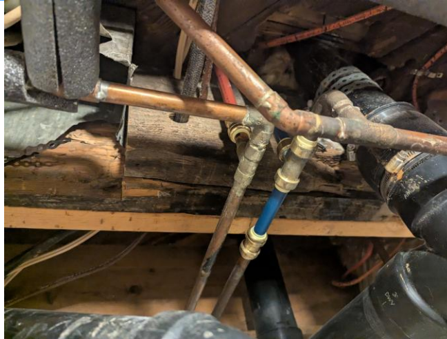
View of the typical copper supply plumbing serving the building.
