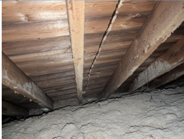
View of the missing intake venting serving the attic space ventilation.
