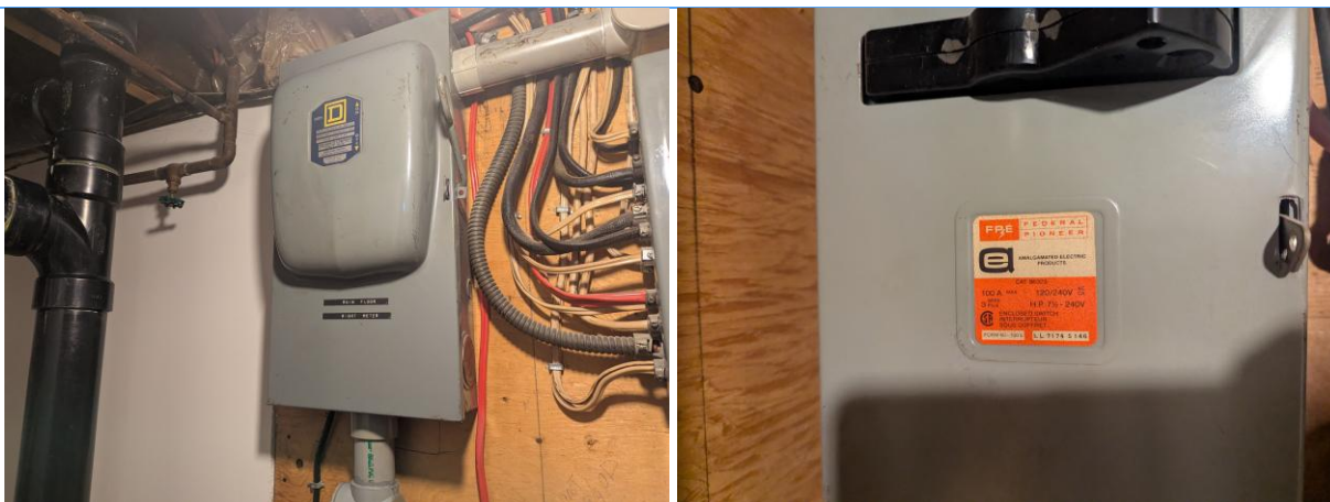
General view of the "Square D" and "Amalgamated" main disconnect switch serving the building.
