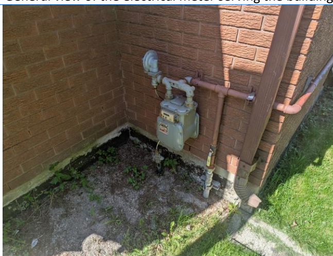
General view of the gas meter serving the building.
