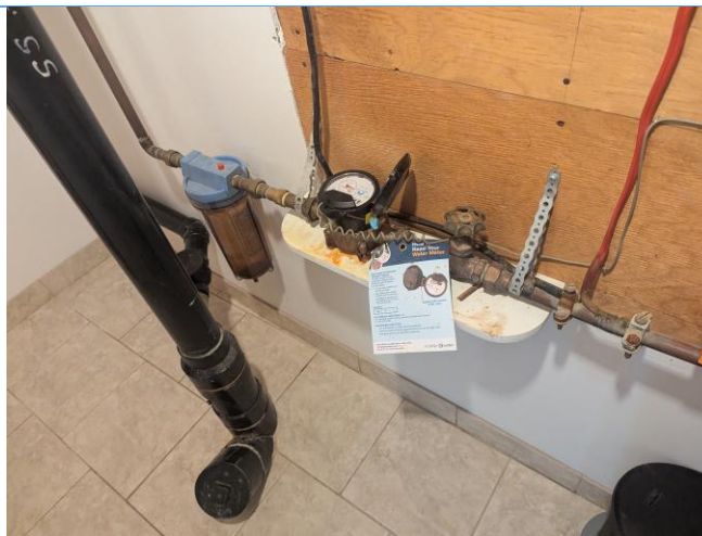
General view of the municipal connection serving the building.
