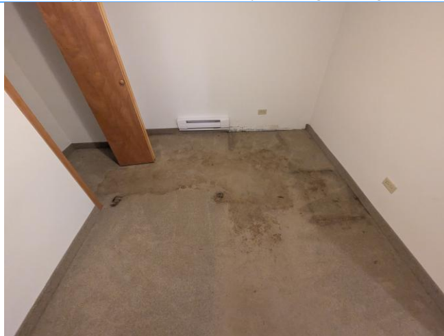
View of the water damage from a previous plumbing leak in Unit 1 basement level.
