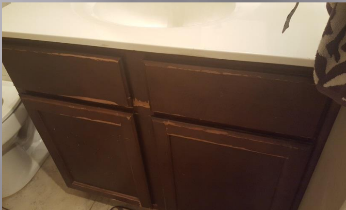
Bathroom Vanity needing paint
