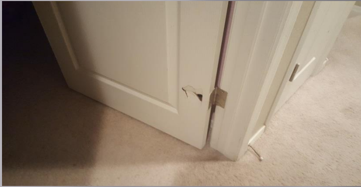
Hole in Bedroom Door
